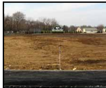
The field is nearing final excavation to prepare for turf installation this Spring.
