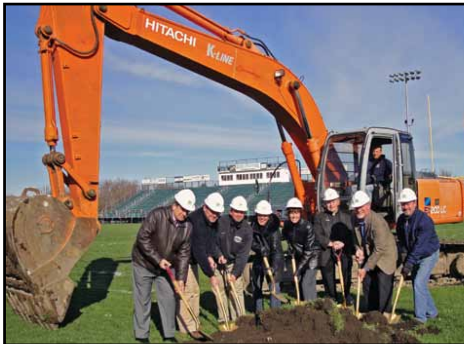
Several members of the PCHS administration and Turf in '12 committee were present at the ground-breaking, which took place in late November. Pictured (left to right) are Donald Sebestyen, Patrick Carr, Doug Ternik '89, Charlie Kaminski, Maureen Harton, Fr. Richard McGrath, OSA, Ed Barrett and Larry Viano.
